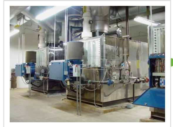
Anaheim Convention Center: 3 WFG-11500 Boilers
