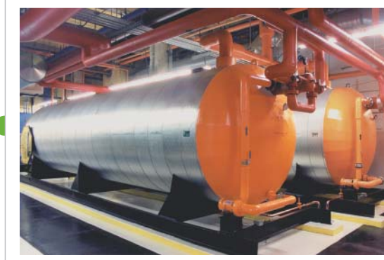
Two 10,000 gallon storage water heaters installed at the San Francisco Marriott Hotel
