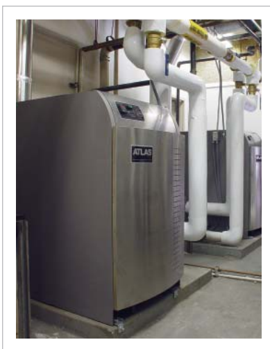
5 Atlas Series condensing boilers installed at the downtown Los Angeles Hilton (Models GS 1.0)
