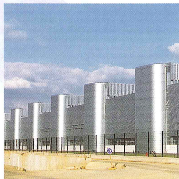
Renault Technical Centre Guyancourt, Paris FAFCO Ice Bank Storage capacity: 46 000 kWh
